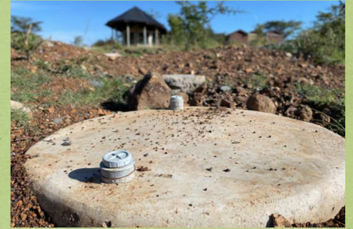
Newly installed biodigester at the Tony Lapham Predator Hub.
